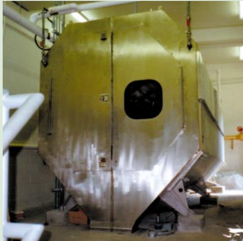
Typical MDS Installation
